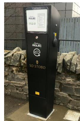
Electric vehicle charging station
