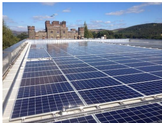
Solar panels on the spa roof
